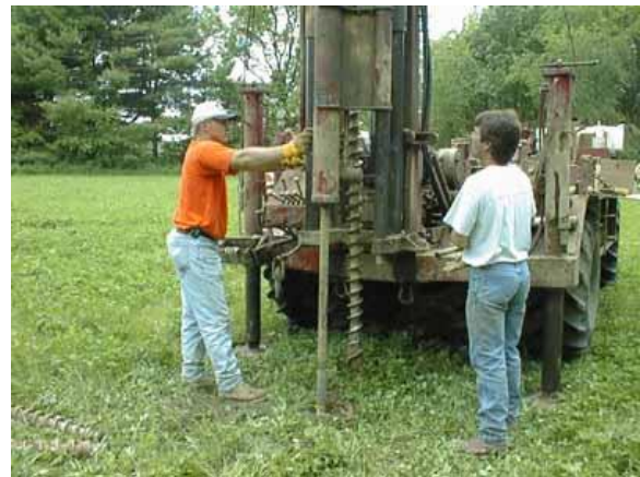
Figure 4. The SPT split-spoon sampler is placed at the bottom of the augered hole. A 140-pound automatic-trip hammer, falling freely approximately 30 inches, drives the sampler a depth of 18 inches. The driller records how many "blows" it takes to drive the sampler each 6-inch increment.
